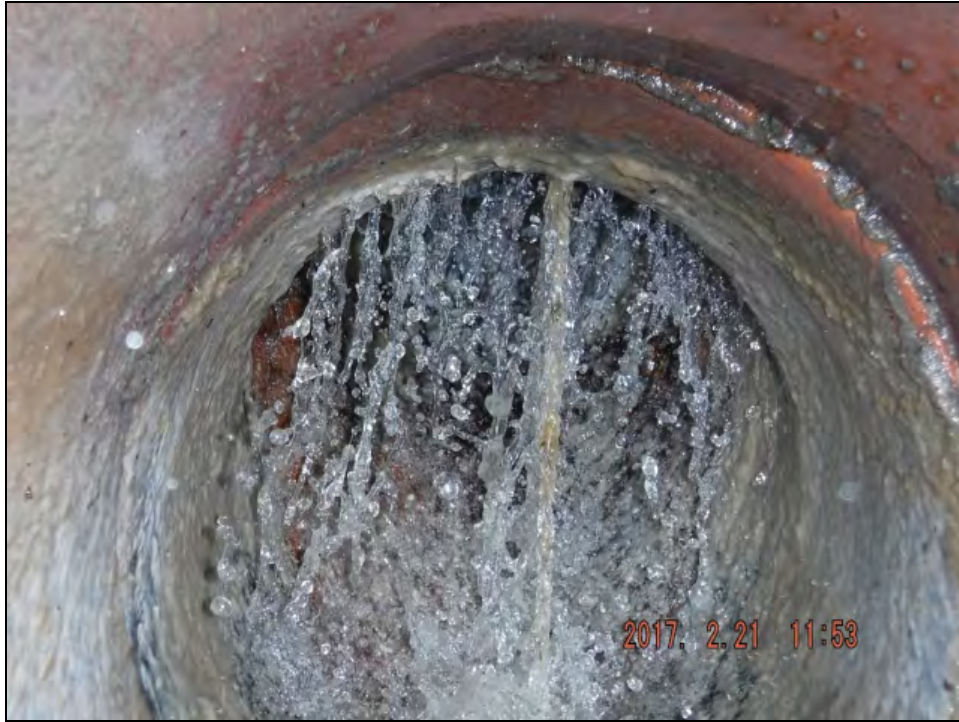
Lower Influent Pipe
