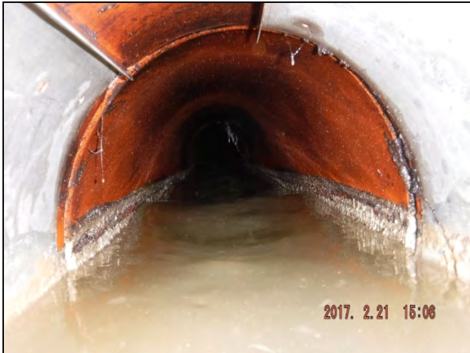
South Influent Pipe
