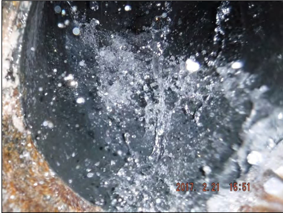
East Influent Pipe (Lower)
