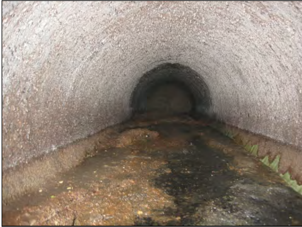
East Plugged Pipe
