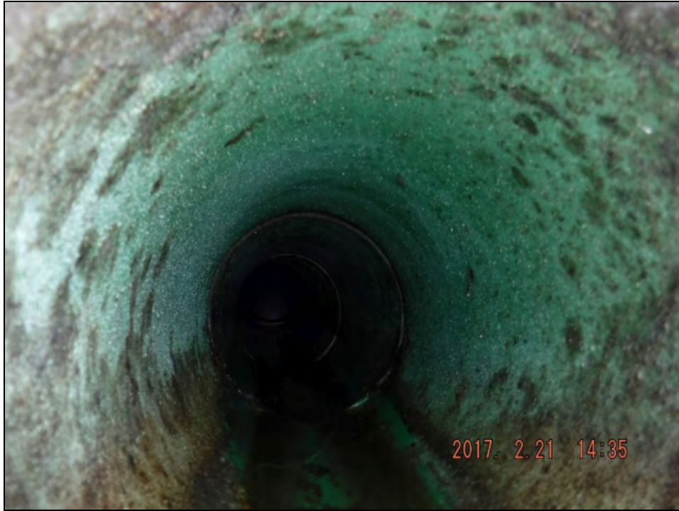
East Influent Pipe
