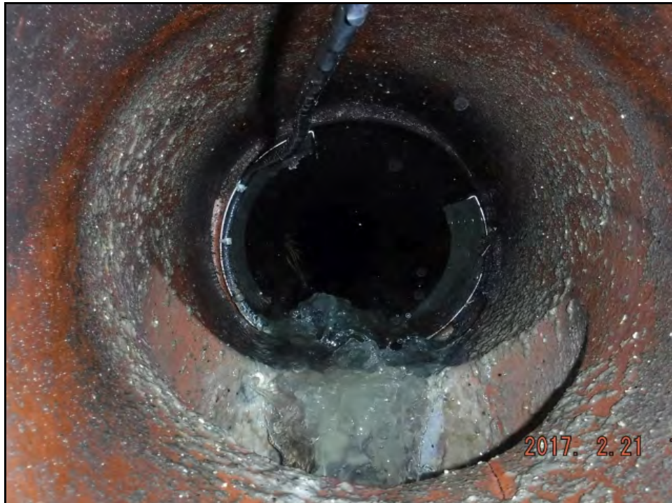
Upper Influent Pipe
