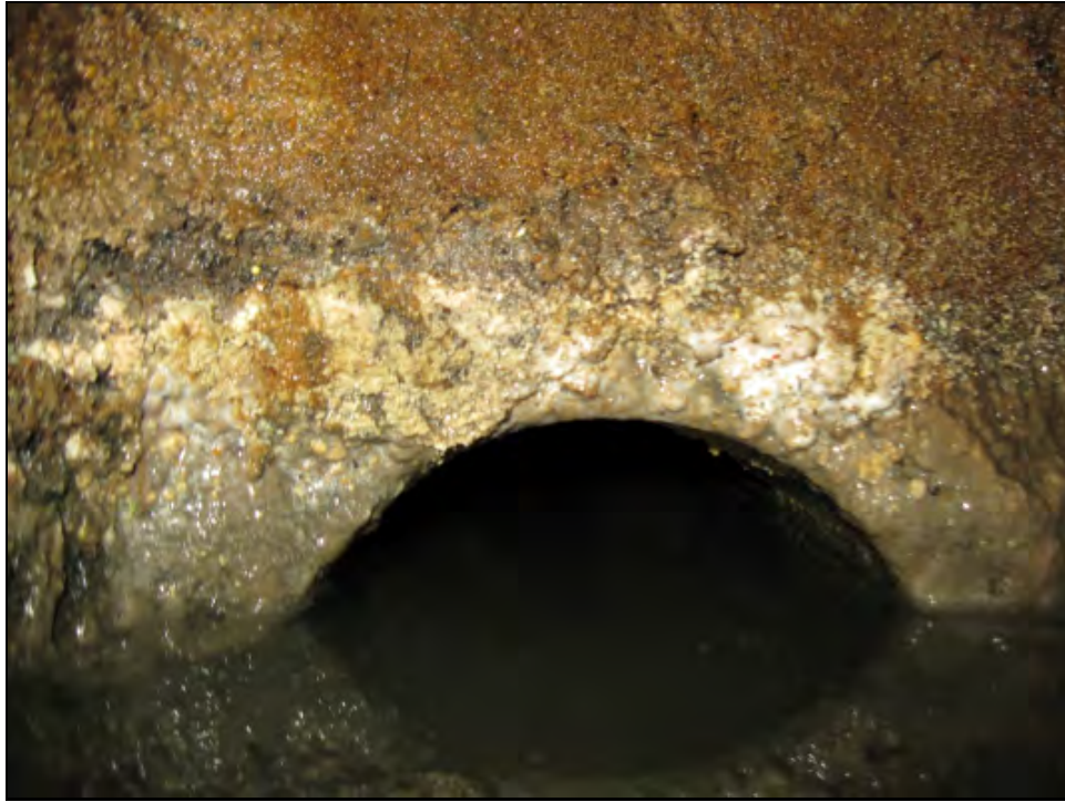
South Influent Pipe
