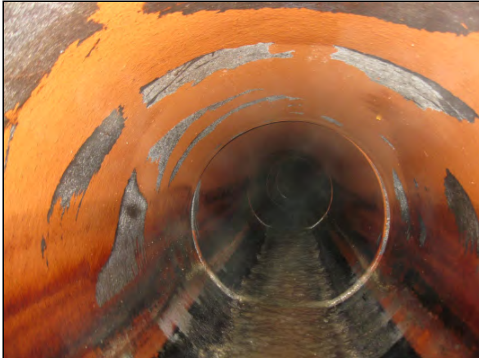
South Influent Pipe
