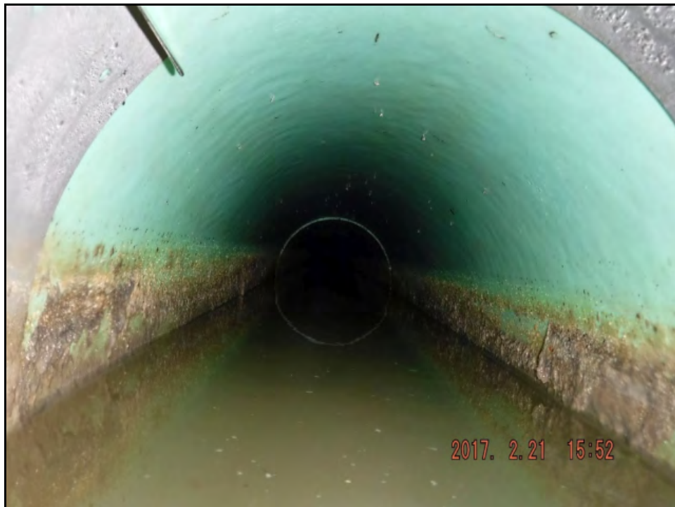
West Influent Pipe
