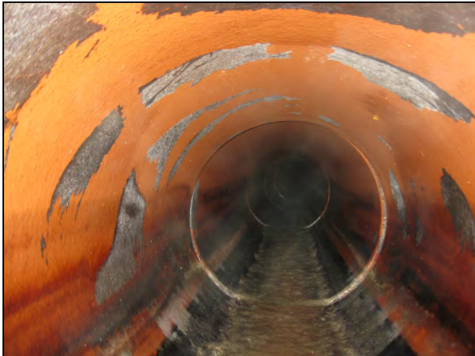
South Influent Pipe
