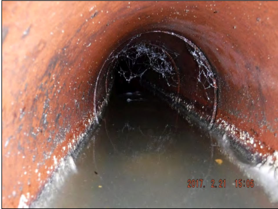
West Influent Pipe
