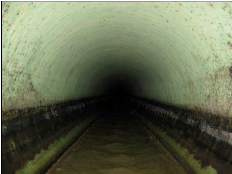
North Inluent Pipe
