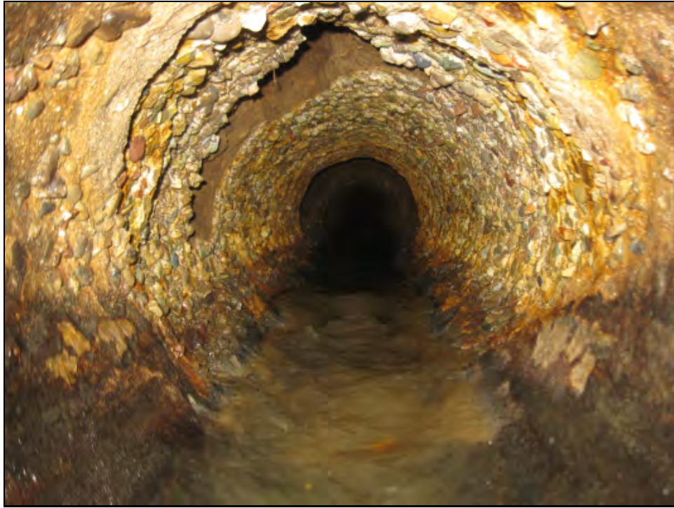
East Influent Pipe
