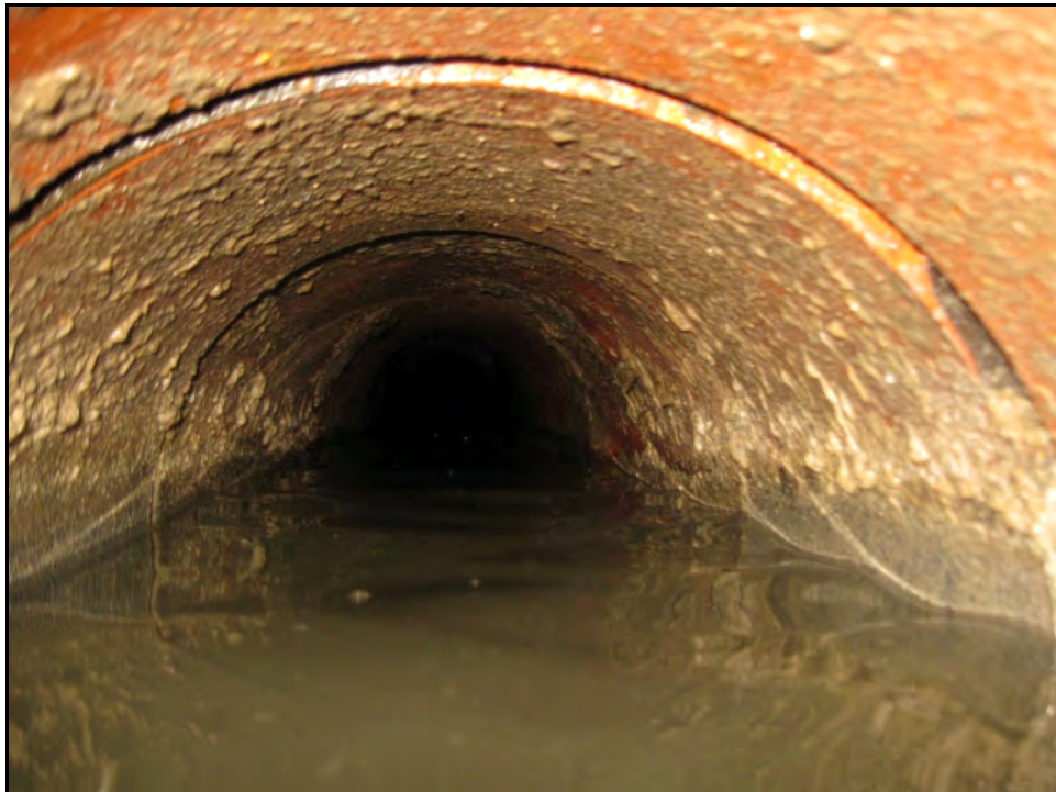
East Influent Pipe
