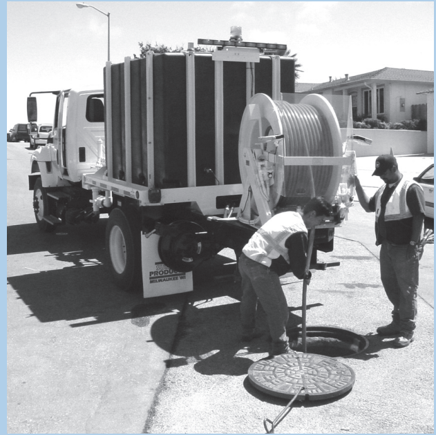
Collection Operator Martin Rosales (right) and System Operator Tuan Nguyen operate the District's new jetter that uses 2,000 pounds of water pressure to remove obstructions, such as grease build-up, from the sewer mains. With 200 miles of sewer mains beneath our streets, the work is ongoing.
