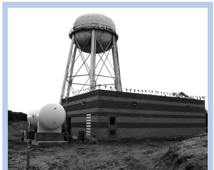
The booster-pump station (foreground) is in the final stage of construction. When completed, it will replace "E" Reservoir (towering behind), which was constructed in 1958, and is scheduled to be demolished next year.
