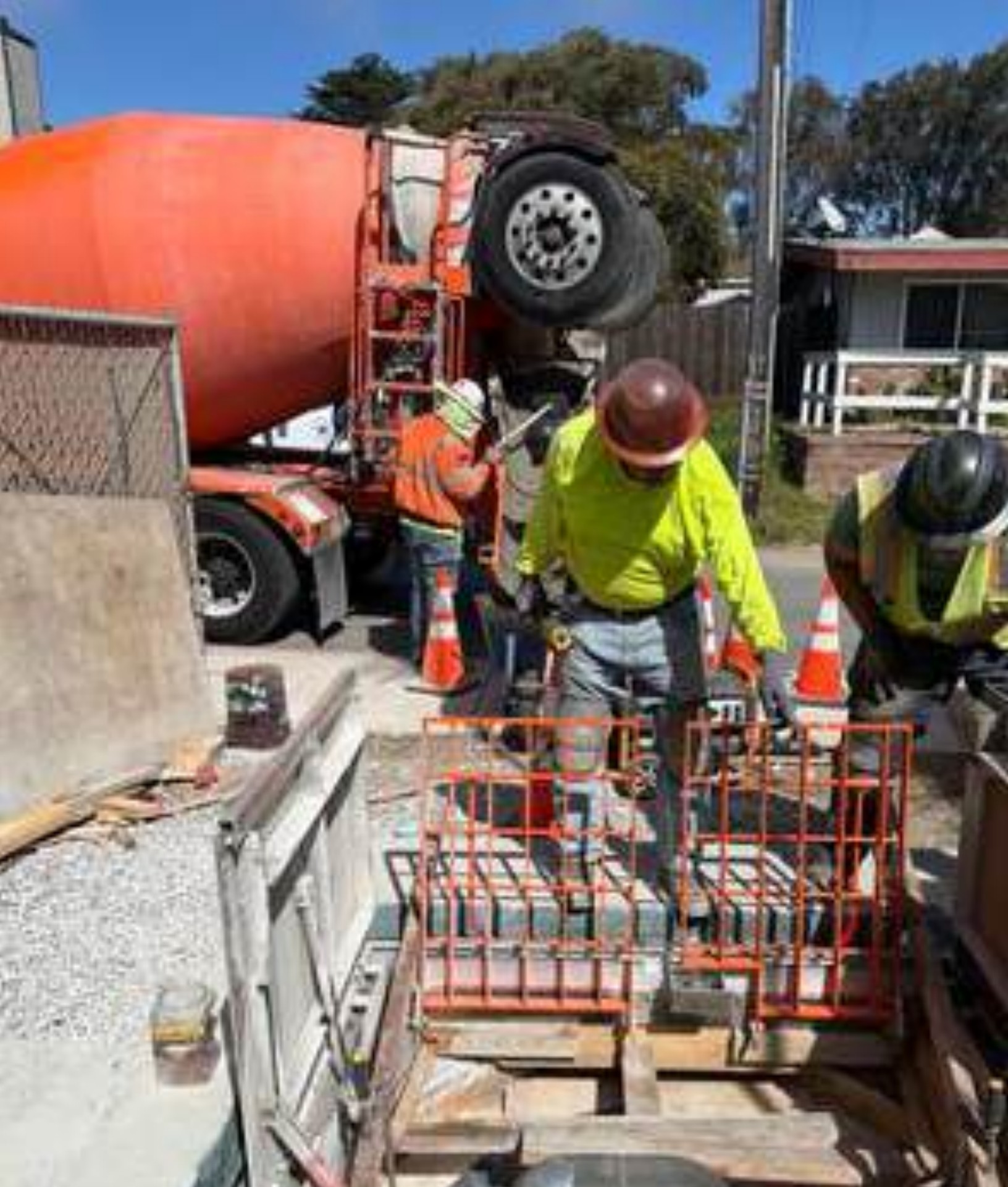
Lift station upgrade in progress—improving reliability, capacity, and long-term performance of the District’s wastewater system.
