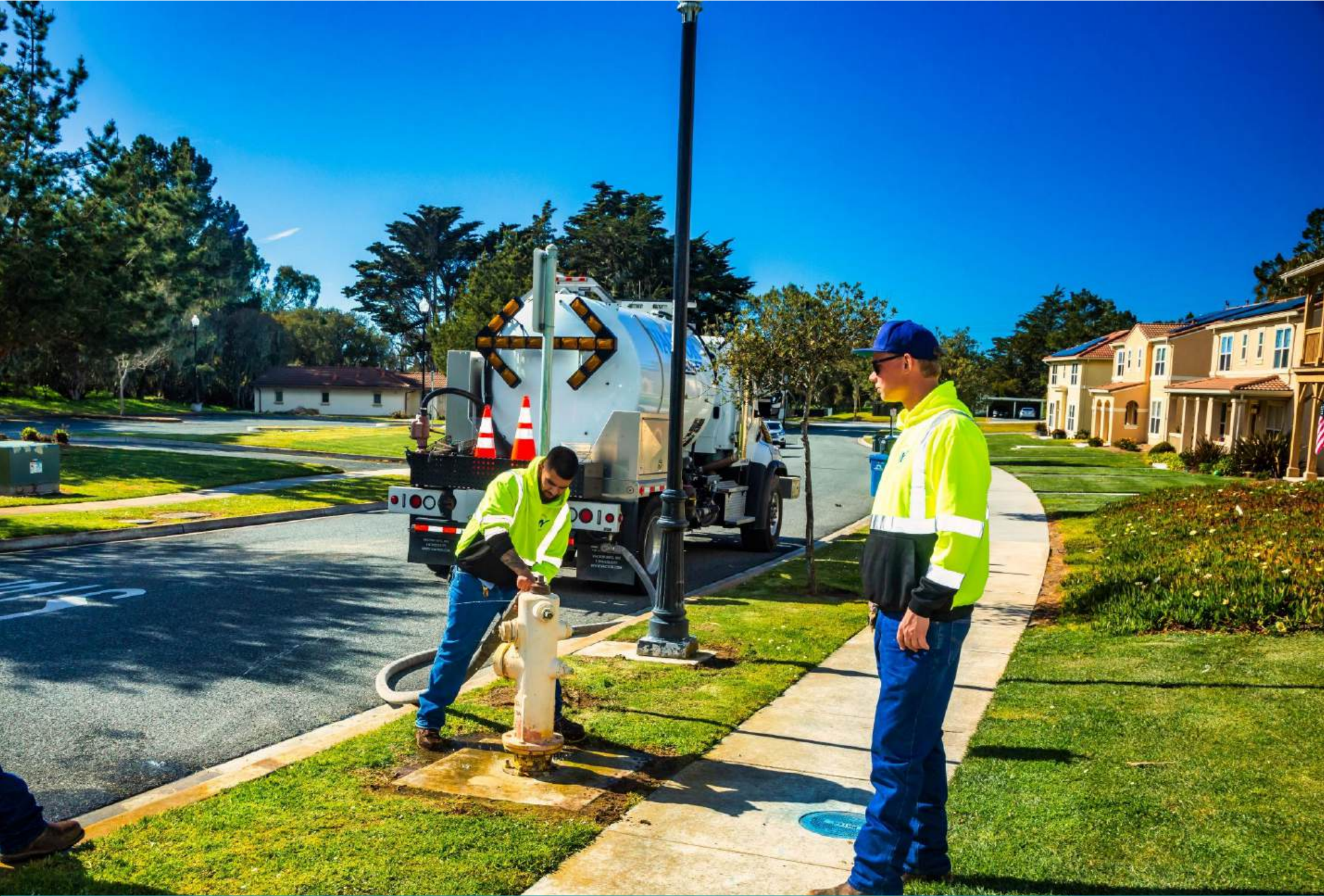
System Flushing—removing buildup and maintaining water quality to ensure safe, reliable service throughout the distribution system.
