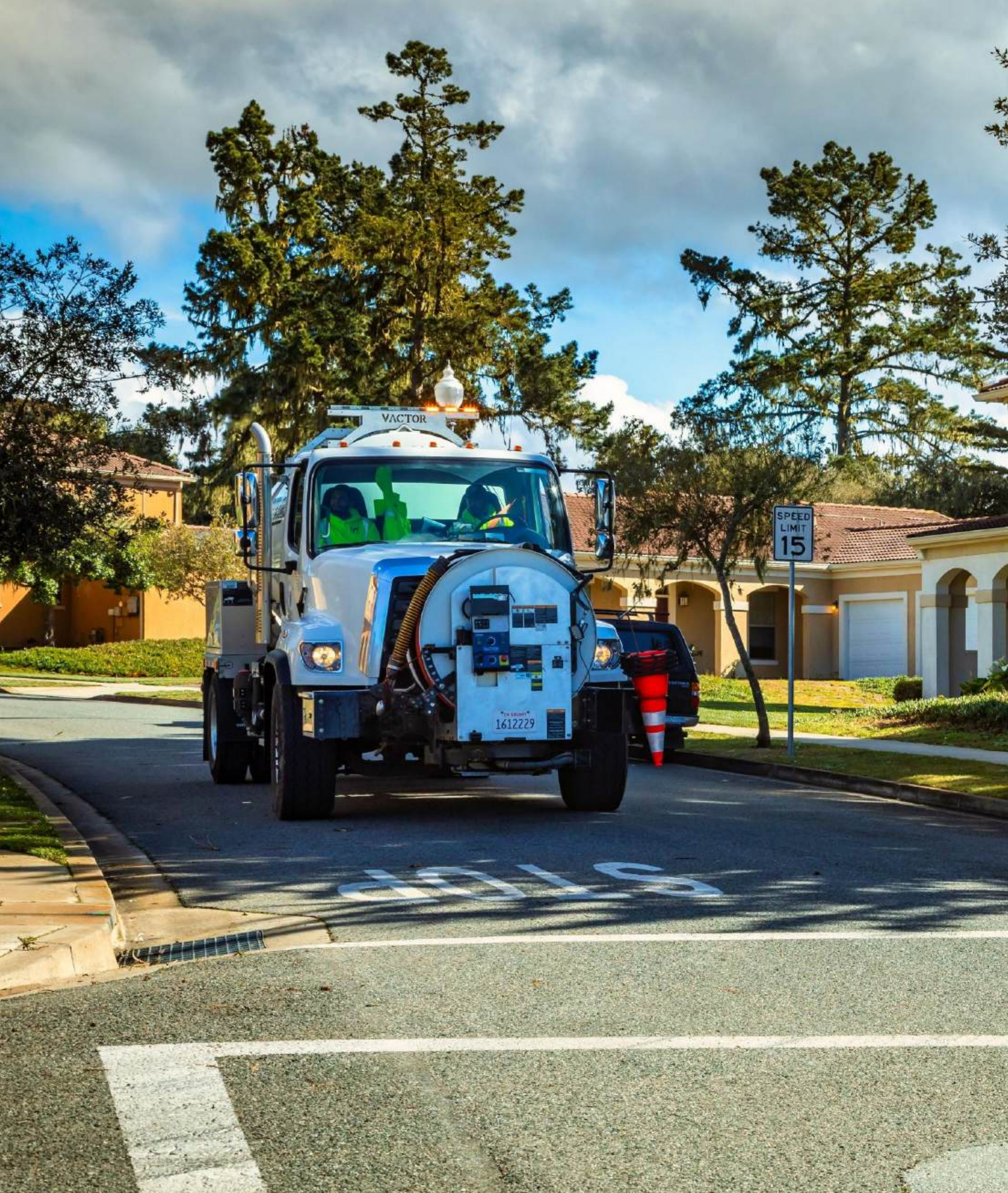
Field crew in action—maintaining and cleaning the system to keep service safe, reliable, and flowing smoothly.
