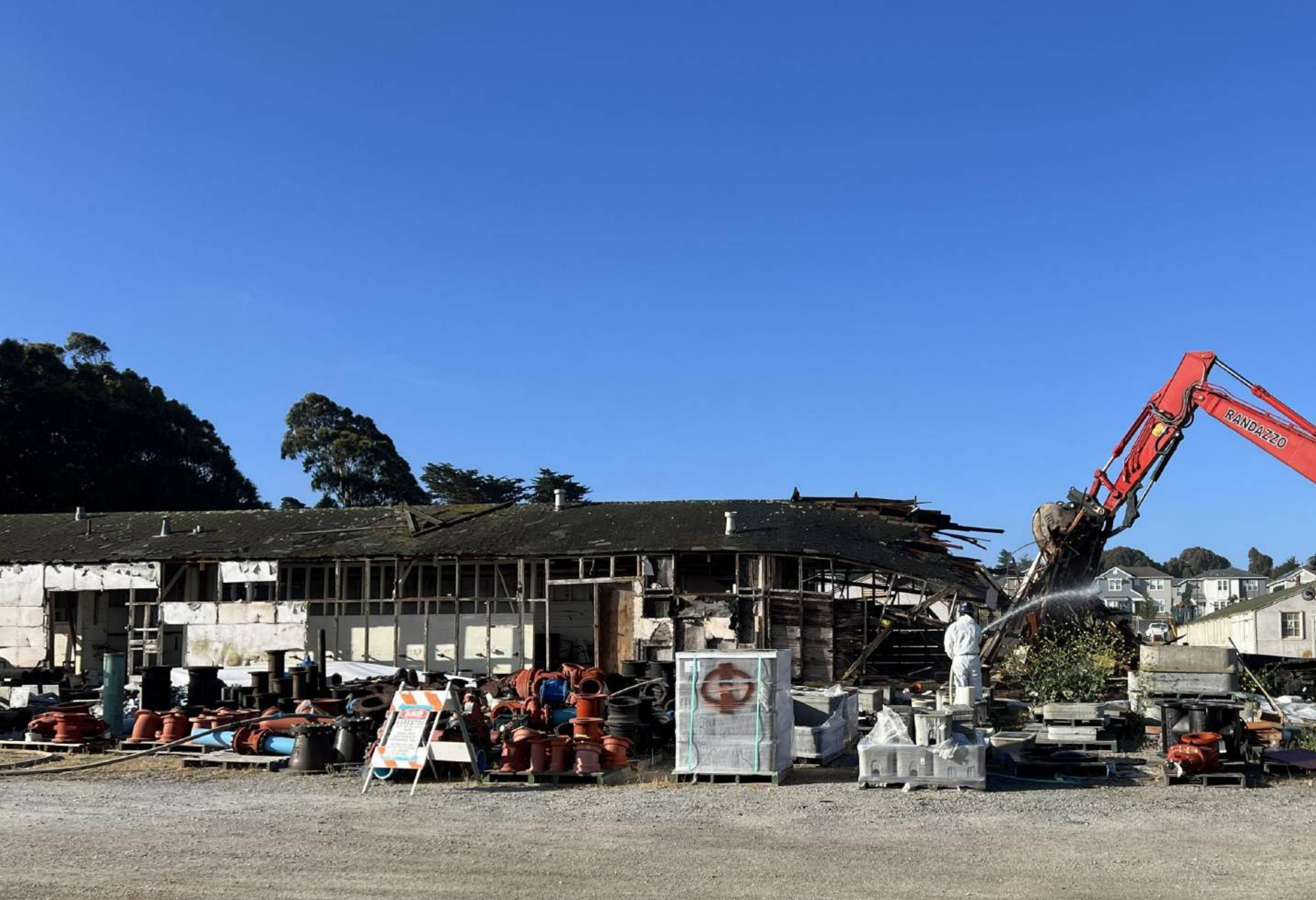
Corporation Yard demolition—clearing outdated structures to make way for future facility improvements and operational upgrades.
